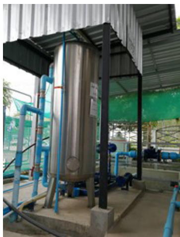
Wastewater treatment system at Nikon Lao Co., Ltd.
