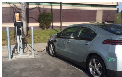
Electric vehicle charging station at Nikon Precision Inc.
