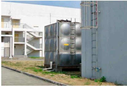
Concentrated water storage at Nikon Imaging (China) Co., Ltd.
