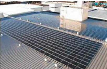
Solar power generation panel at the Kumagaya Plant
