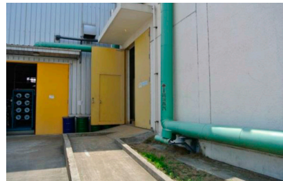
Steam pipes running inside the premises at Nikon Imaging (China) Co., Ltd.
