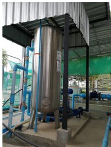
Wastewater treatment system at Nikon Lao Co., Ltd.
