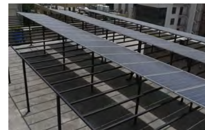
Solar panels installed at Nikon India Private Limited
