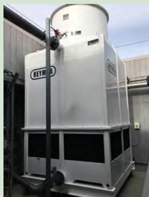
The new cooling tower at Nikon Precision Inc.
