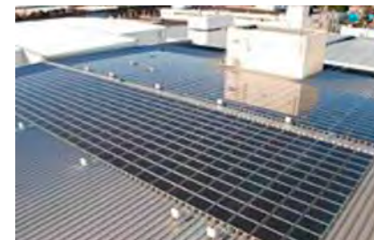
Solar power generation panel at Nikon Kumagaya Plant
