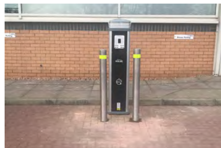
Electric vehicle charging station at Optos Plc
